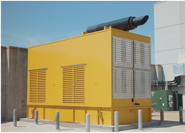
Exhibit 9. EPS Located in Heated and Secured Outdoor Enclosure. Note that the area is not subject to flooding. ( Courtesy of the International Association of Electrical Inspectors )
