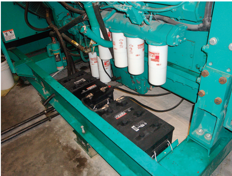
Exhibit 11. Detail of Batteries Used for Starting Engine Used for Emergency Power. Note the clean contacts.
