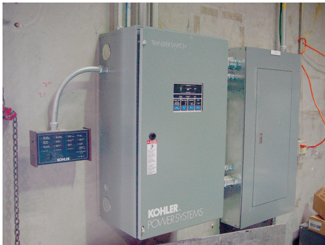
Exhibit 4. An Emergency System Transfer Switch. (Courtesy of the International Association of Electrical Inspectors)
