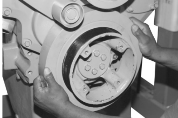
Checking Damper Rotation
