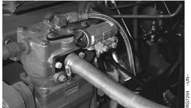
Inspect Air Compressor
