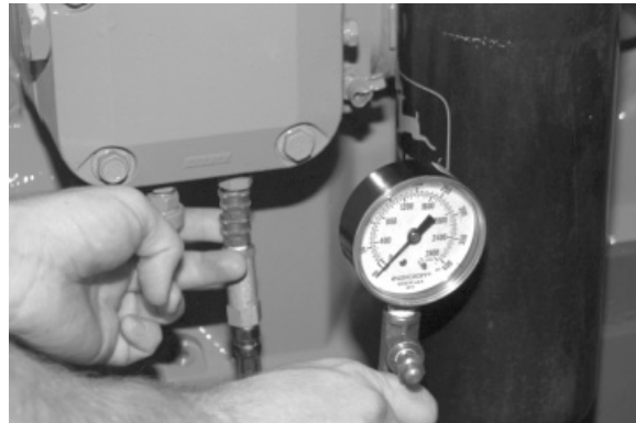
Oil Pressure Gauge at Quick Disconnect on Oil Cooler
