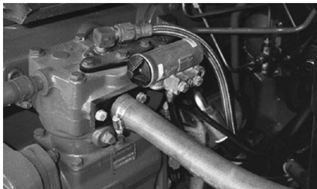
Inspect Air Compressor (Midland Compressor Shown)
