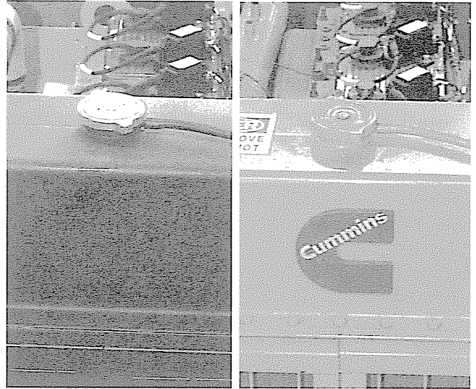
Photo #5-03 - Radiator & Expansion Tank Caps
