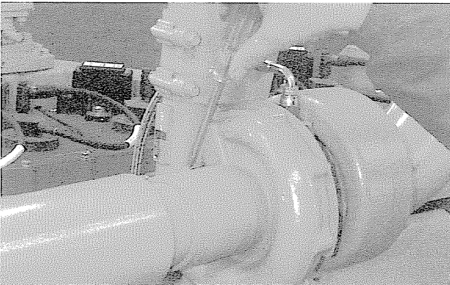
Photo #5-02 - Air Connections
