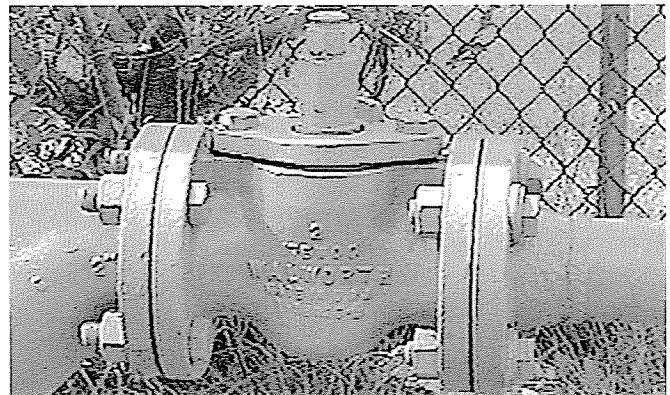
Photo #3-01 - Manual Gas Shut-Off Valve
