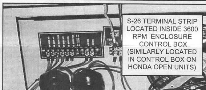
S-26 ALARM INTERFACE APPLIED TO THE 3600 RPM ENCLOSURE CONTROL BOX
