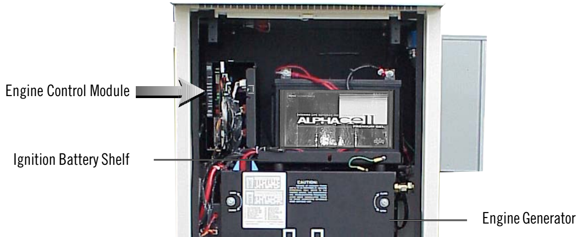
Fig. 1-4 Location of Engine Control Module within the Engine-Generator Cabinet.
