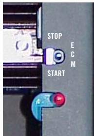
Fig.2-2 Generator Control Board master switch
