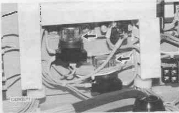
Magnetic Switches Location
