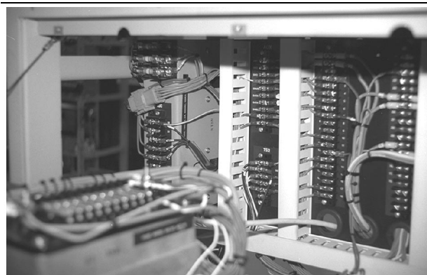
Illustration 87 g00619154 Terminal Strips (Control Panel interior)
