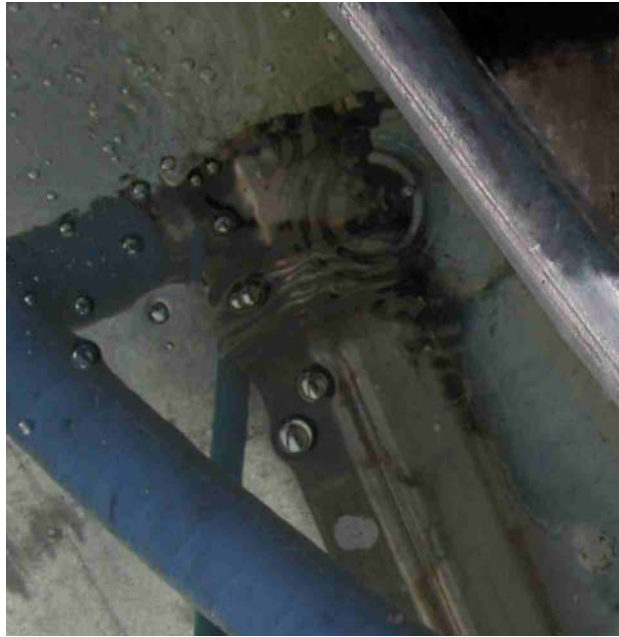
Figure 4 – Stream of air bubbles coming out of the pressurized EGR Cooler
