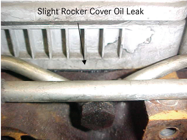
Figure 6. Rocker cover oil leak.
