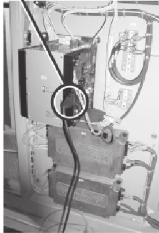
SD70ACE AND SD70M-2 EMDEC ACCESS PORT
