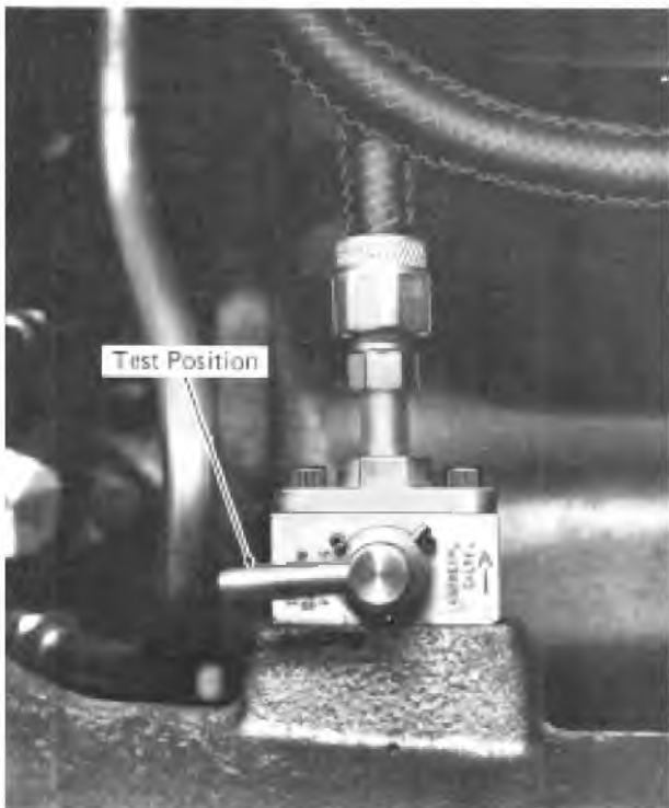
Fig. 13-5 - Test Valve Positions
