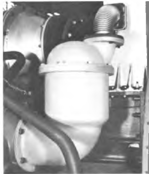
Fig. 9-10 - Lube Oil Separator
